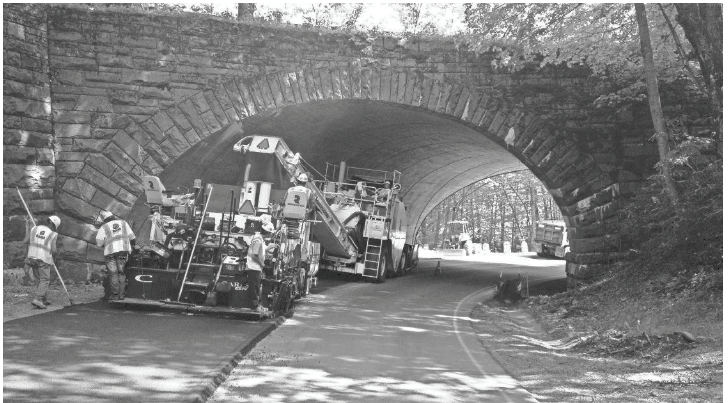
Great Smoky Mountains National Park maintains and operates more than 300 miles of roads, six tunnels and 146 bridges. Road paving, such as that shown here on Newfound Gap Road, will be part of deferred maintenance addressed by funds provided by the Great American Outdoors Act. COURTESY PHOTO
