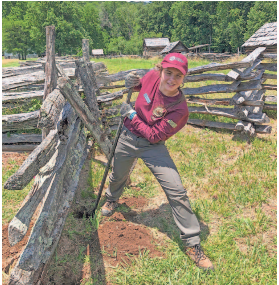
Great Smoky Mountains National Park summer intern Phoebe Carnes of Whittier struggles to loosen a large underground rock with a pry bar while repairing a fence at the Oconaluftee Visitor Center. PHOTOS PROVIDED BY NATIONAL PARK SERVICE
