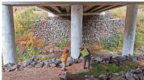
Ben Prater, right, and Tracy Davids of Defenders of Wildlife spot animal tracks under Harmon Den Bridge. This dirt path was installed as a more wildlife-friendly alternative to riprap, encouraging animals to cross safely underneath the interstate.
