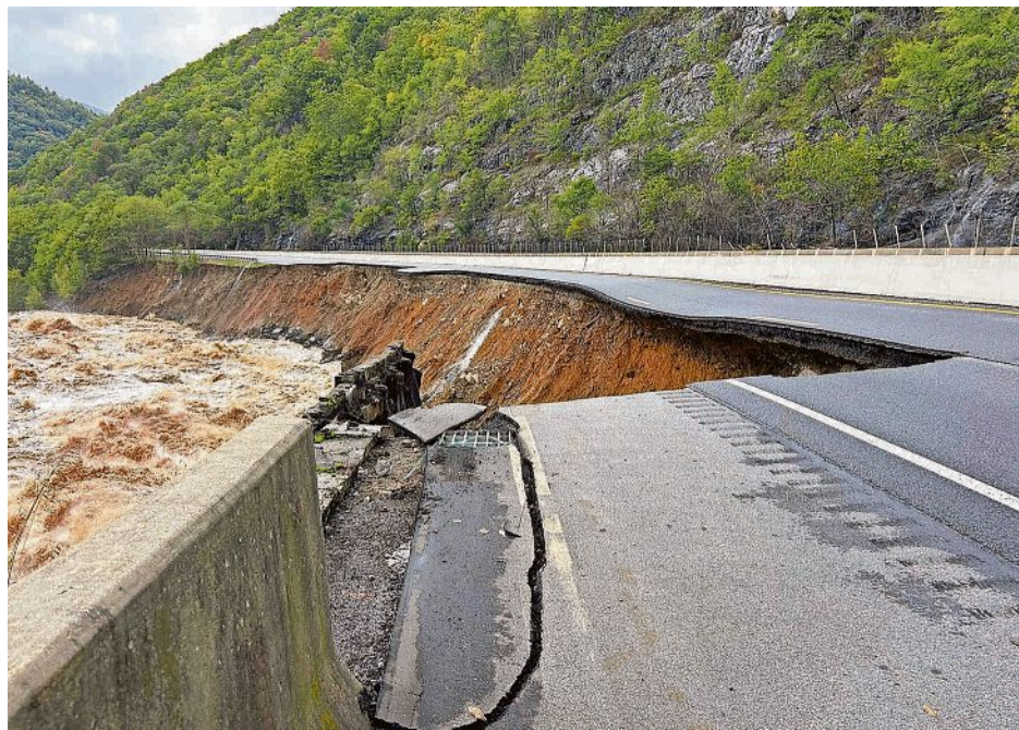
Following Hurricane Helene, eastbound lanes of I-40 had collapsed into the Pigeon River over much of a 4.5-mile stretch extending from the double tunnel to the Tennessee-North Carolina line. PROVIDED BY NCDOT
