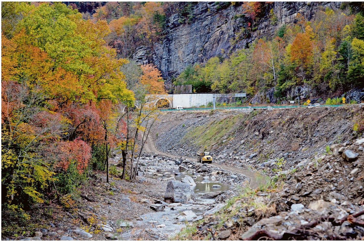
NCDOT crews engage in preliminary road work ahead of the final plan's release and implementation.
