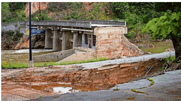
The Gashes Creek Road Bridge at Recreation Park in Asheville on May 16, 2025.
